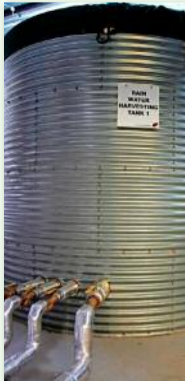
30,000 litre storage tank holding rain harvested water to feed the plate cooler in the new dairy unit at CAFRE, Greenmount.
